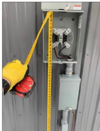
Meter installed 3 feet 6 inches to 5 feet above final grade.
