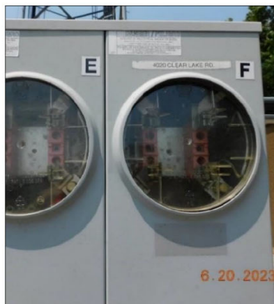
Multiple meter labelling. Meters must be labelled with address or unit number.
