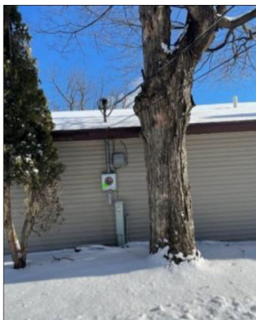
Approved overhead service, meter set only.
