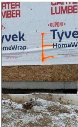
Meter location marked.
