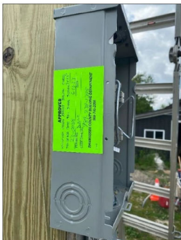
Meter socket inspection sticker.
